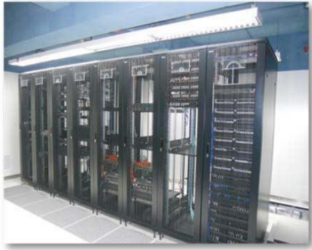
A dedicated data center or a functional area within
